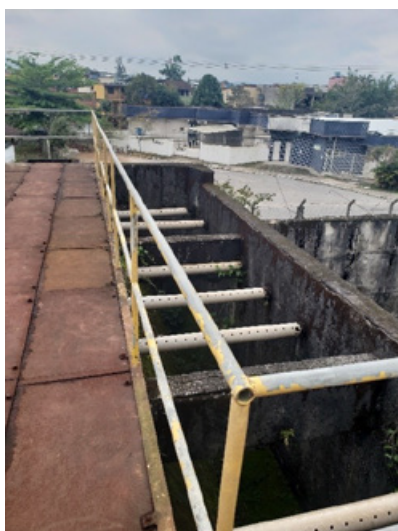
FIGURA 6-55 – ETE FRADE – REATOR UASB – VISTA SUPERIOR
