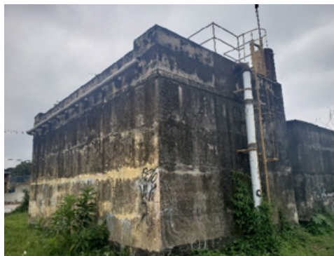
FIGURA 6-54 – ETE FRADE – REATOR UASB
